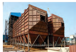
Air Pollution Control Equipment
