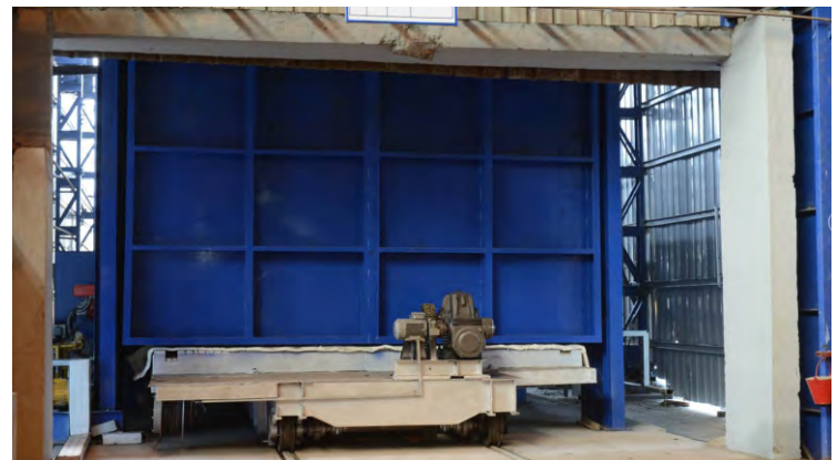
Heat Treatment Furnace
