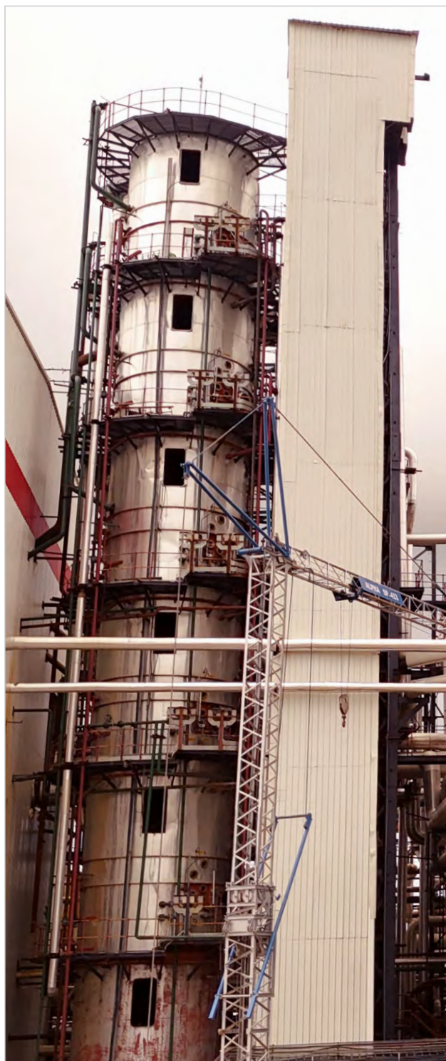
45 TPH VCP at Bindal Paper Mills Ltd., India
