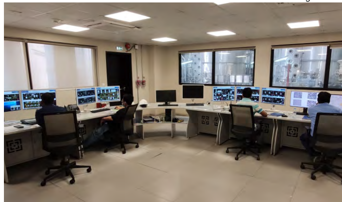
Centralised Control Room for a Sugar Plant
