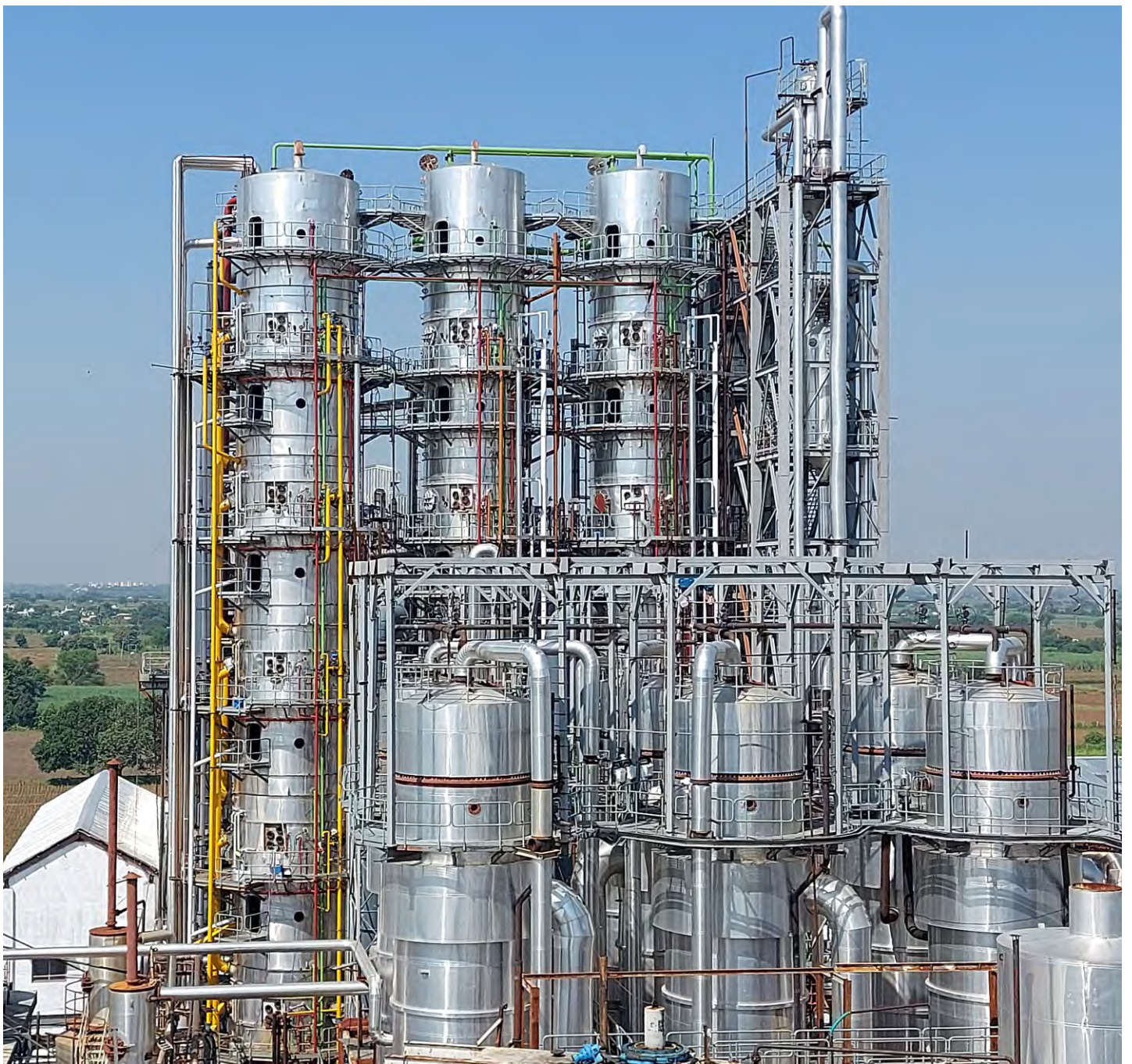
3 Nos. VCP at Twenty One Sugars
