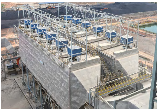
67.5 MW CFBC Power Plant at Bhubaneswar Power Pvt. Ltd., Bhubaneswar
