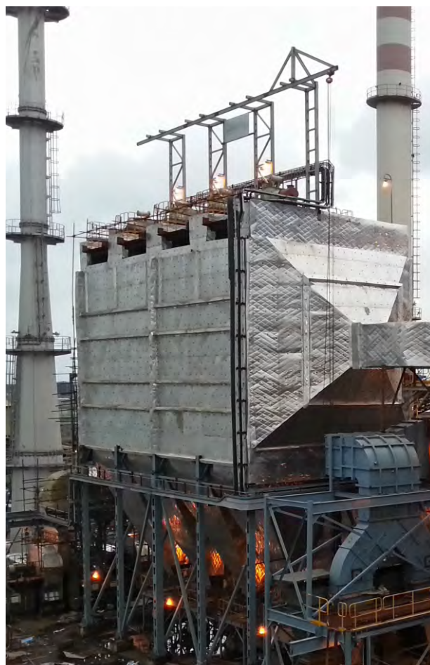
22 MW AFBC Power Plant at Gujarat Fluorochemicals Dahej, Gujarat
