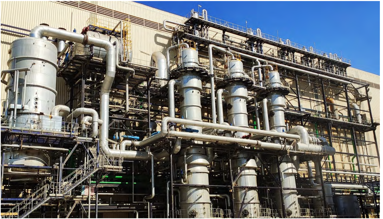
2500 TPD Standalone Refinery - Triple Effect Mill Concentrator Falling Film Evaporator at Durrah Advanced Development Company, Yanbu Port, Saudi Arabia
