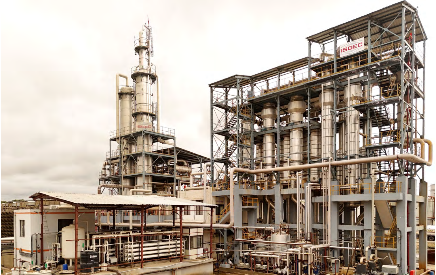
120 KLPD Ethanol Plant with 25 TPH Incineration Boiler & 2.5 MW Cogen Plant Multi-Feed Syrup / B Heavy / Grain at Bindal Papers Ltd., (U.P.), India
