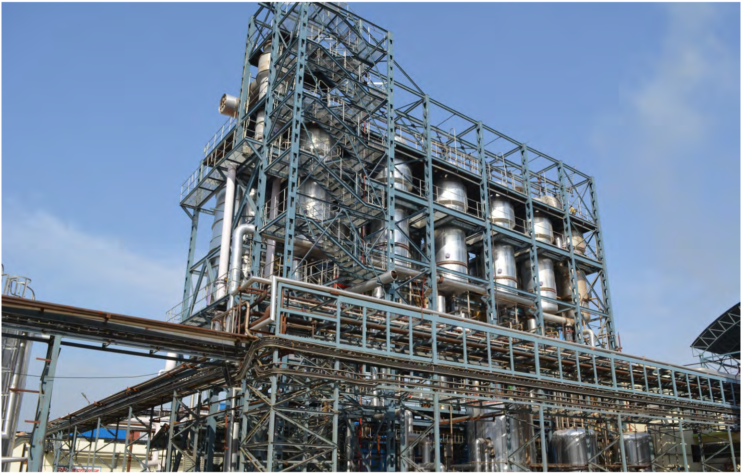
130 KLPD Distillery Plant at Dwarikesh Sugar Industries Ltd., Bijnor (U.P.), India
