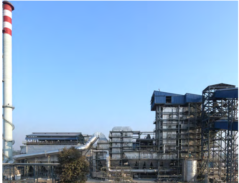
80 TPH, 45 kg/sq.cm. (g), 400 Deg. C, Slop / Bagasse Fired Travelling Grate Boiler at DCM Shriram Sugars, Ajbapur (U.P.), India
