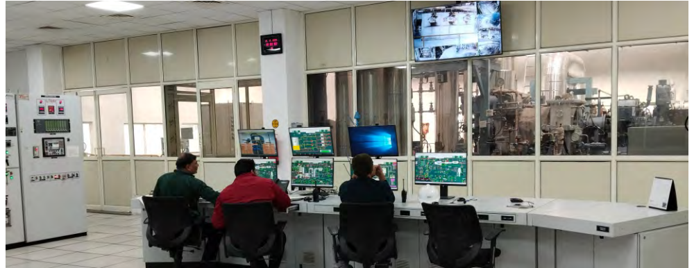
Centralised Control Room at a Distillery Plant
