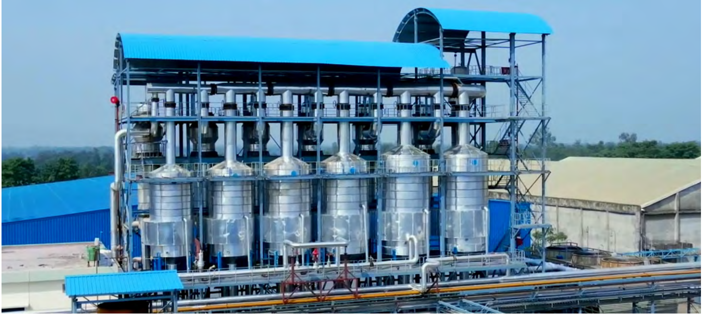
Spent Wash Evaporator System for 175 KLPD Ethanol Plant at Dwarikesh Sugar Ltd., (U.P.), India
